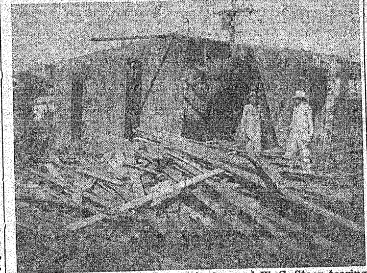
PICTURED ABOVE is Bert Howington and W. S. Stacy tearing down an old land mark in Santa Anna that everyone is glad to see gone. The building was the old house on Avenue B, in front of the North Side Baptist Church. The lot has now been cleared off and all rubble burned.
