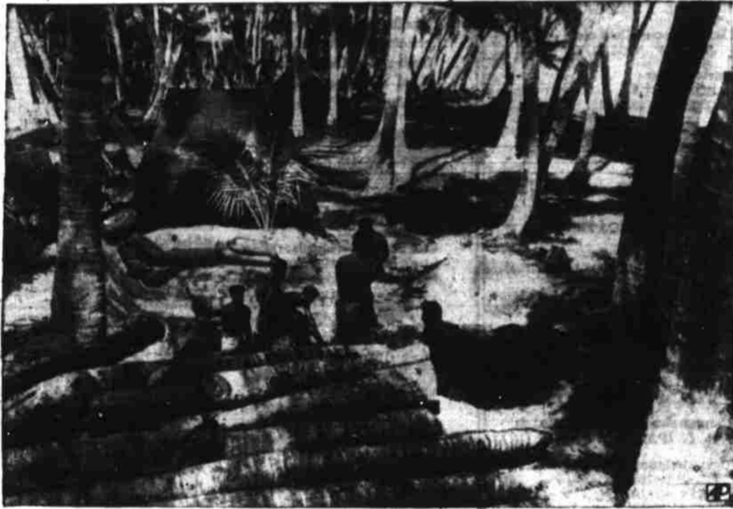
CONSTRUCTION GANG —A gang of native laborers excavates for a command post at one of the advanced bases of the 7th USAAF somewhere in the Gilbert Islands.
