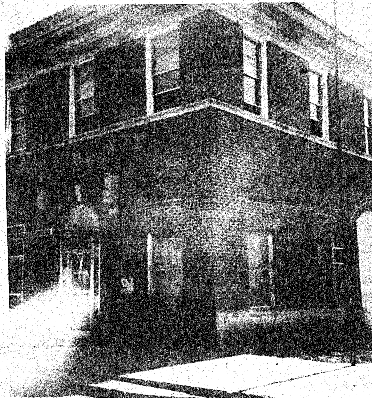
THE CITY HALL AND FIRE DEPARTMENT BUILDING received a sort of facelift this week with the replacement of windows. The project is a joint effort of the Fire Department and the City of Santa Anna.
