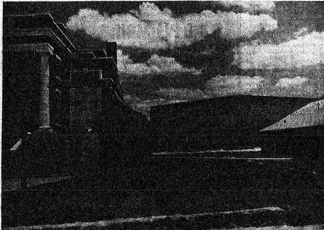
WORK IS CONTINUING on the Christian Life Center at First Baptist Church. The exterior work is almost completed for the large building that will contain offices and rest rooms, a nursery, classrooms, a
