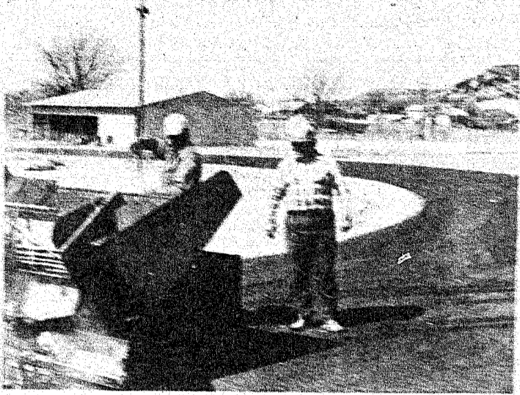
WORKING ON TRACK —Derral Warnock, Booster Club President, looks on as work was in progress on the new Donham Memorial Track at the school stadium. Warnock was instrumental in the planning and completion of the project that was a joint effort of the Booster Club and the school.
