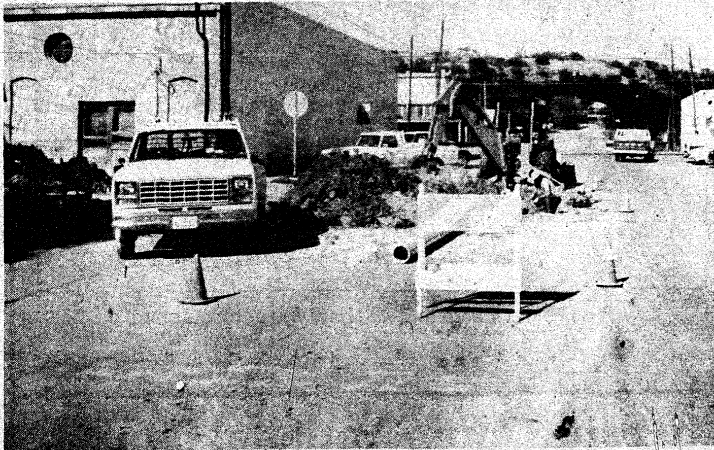
CONSTRUCTION IN PROGRESS in the downtown area is for replacement of gas lines that have been in use as long as 65 years. Lone Star Gas Co. expects the main work to be completed this week, with Earl Deen Plumbing
