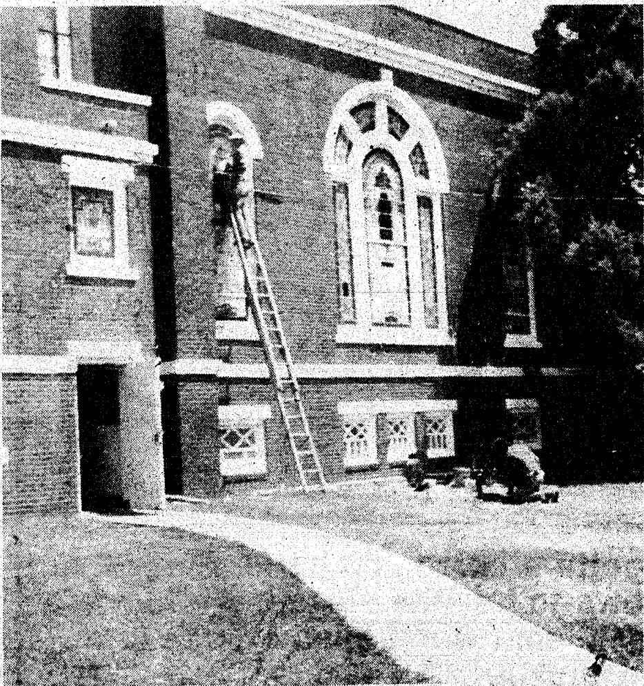
WORK IS IN PROGRESS at First Baptist Church on the stained glass windows, with workers from the Hauser Studio of Stained Glass of Winona, Minn. doing the work. Jack Chap (atop ladder) and Pat Flannigan will be working through next week re-leading and painting the windows and installing a transparent covering for protection from hail or vandalism. The project will cost over $13,000 and is being financed by donations and memorial gifts. The 32 stained glass windows have been valued at over $90,000. The church was built in the early 1920s.
