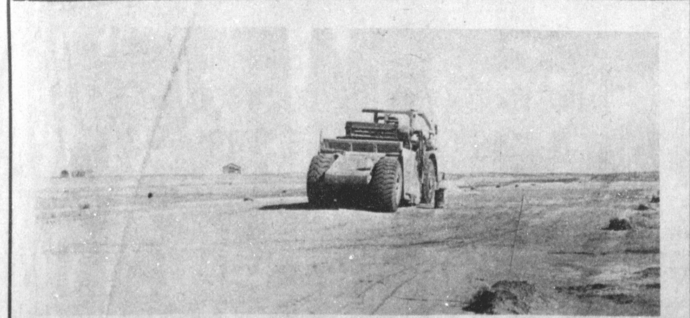
LOTS OF DIRT BEING MOVED AROUND--At the site of the new city airport east of Muleshoe, land is being leveled and stakes are being set out to define future runways. Dirt work is preliminary to building hangars, runways, access roads and everything else that goes with a brand-new airport. Laying the surface of the new runways is expected to start sometime in the next few months, although final construction at the site won't be completed for several months yet. Caprock Construction of Lubbock is the general contractor who won the bid for construction of the new airport.
