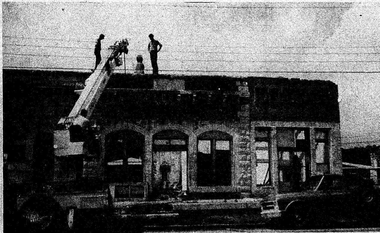
LANDMARK BEING MOVED. The three old buildings located on main street are being torn down for a move to Salado, Texas, where they will be re-constructed in that historic town. Workmen are shown here moving the rock coigns from atop
