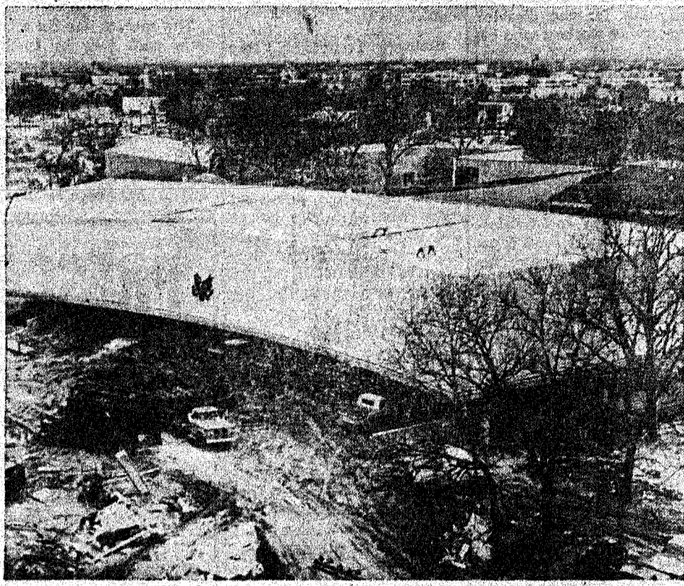
UNITED STATES PAVILION—Work on the exterior of the United States exhibit hall, one-half of a $6.75 million pavilion complex at HemisFair '68, nears completion and attention is turned to the interior design. This picture of the structure, marked by the United States Seal, was taken atop the Swiss Skyride already in operation at the San Antonio World's Fair.
