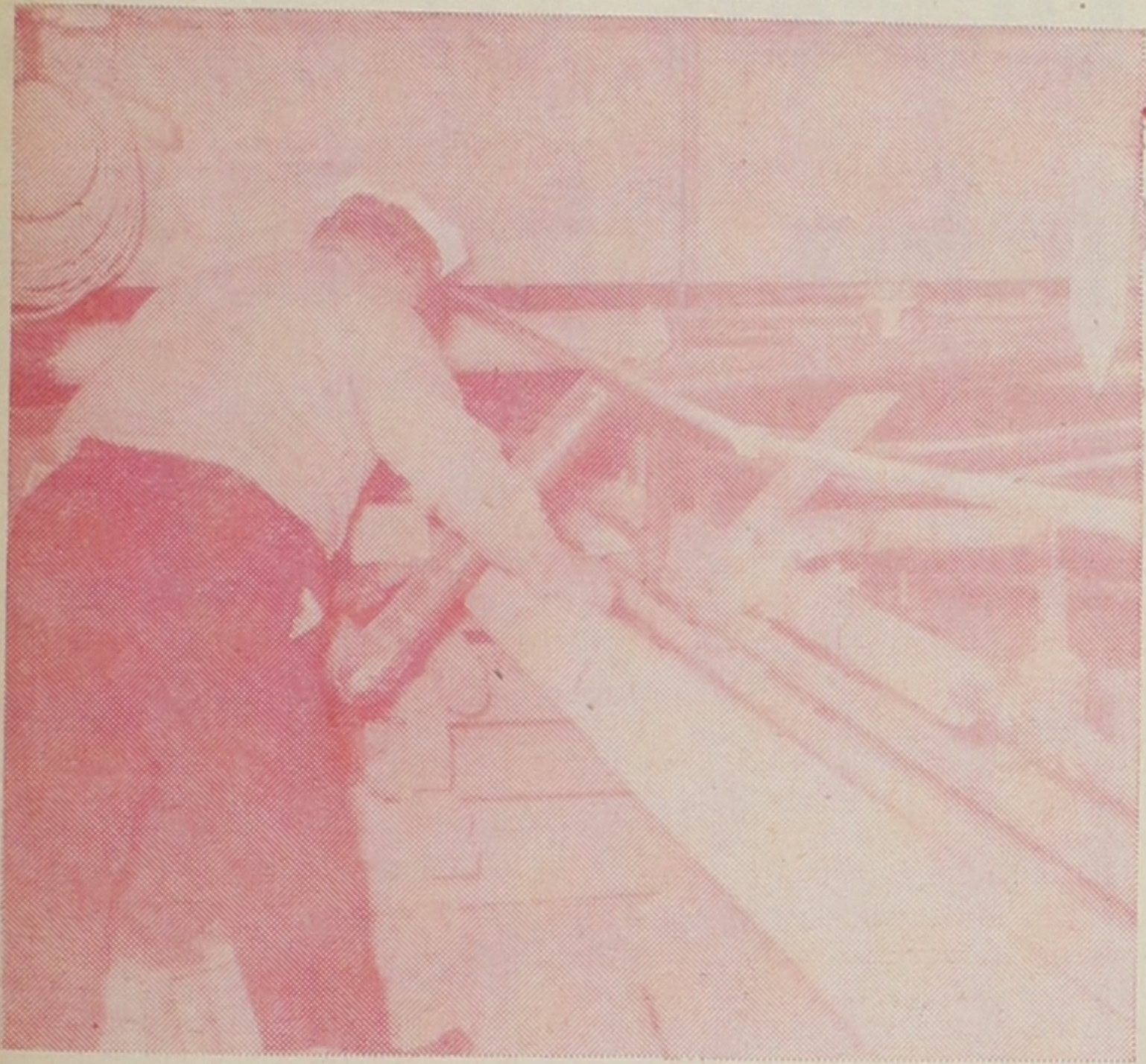
SMOKEY PIPES — A misplaced coated steam pipe (arrow) in the basement of the Ad Bldg. under room 116 brought nine units and 26 men from Stations 1 and 4 of the Lubbock Fire Dept. scurrying to the Tech campus at 3:10 p.m. Friday. The "fire" turned out to be smoke from excessive heat liberated by the melting pipe coating. The alarm was turned in by Don Renner, assistant registrar.
