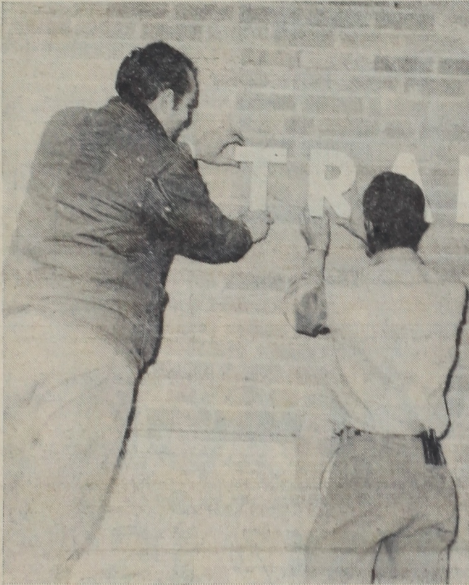
SIGNS OF CHANGE — The buildings on Tech campus have acquired a new look with the addition of signs to identify them. Here, workmen are finishing the sign on the Traffic Security Bldg.
