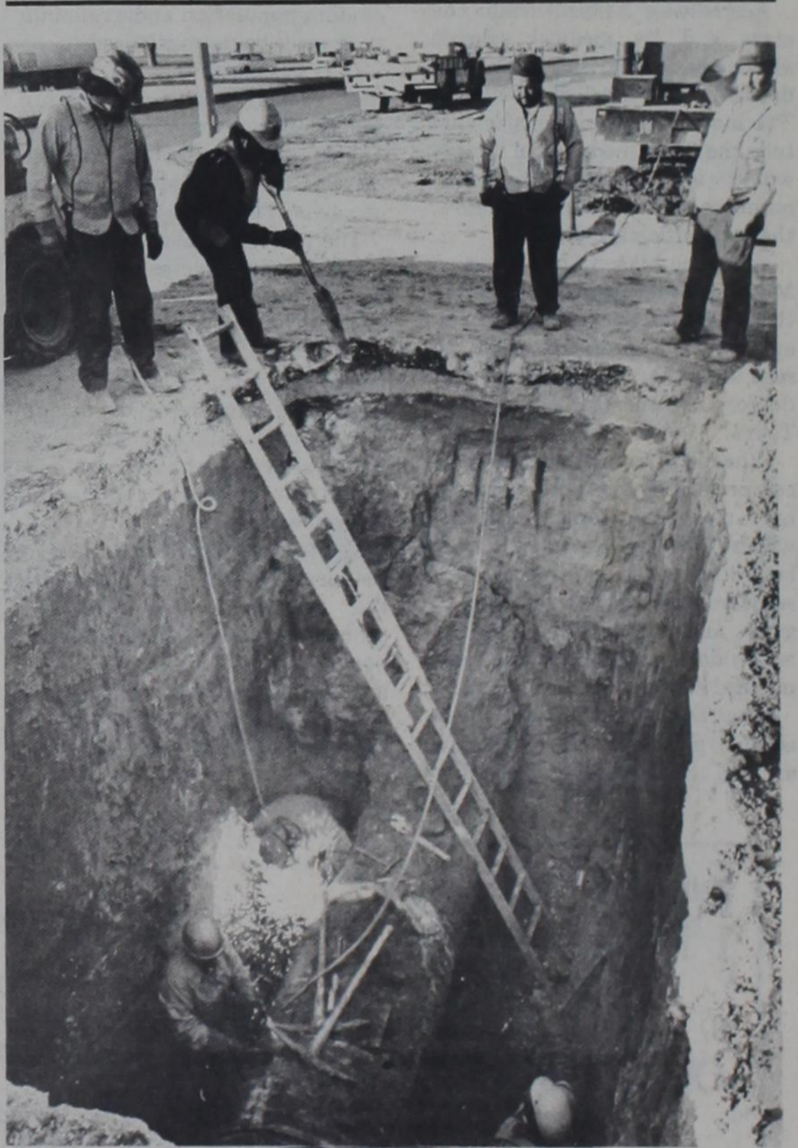
A leaky water main at 19th and Indiana caused traffic to back up four blocks. Repairmen attempt to halt the leak with a welding torch. (Photo by Mark Rogers)
