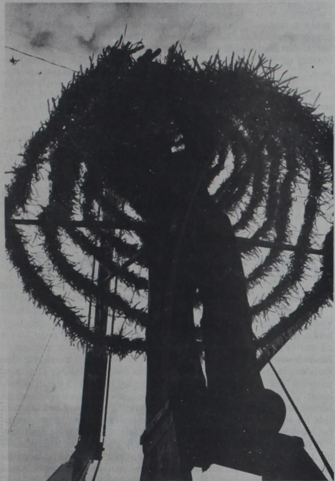
Christmas is fast approaching, and the city is beginning to be decorated for the holidays. Don Ham, Lubbock city employee, prepares the lights along Broadway.
