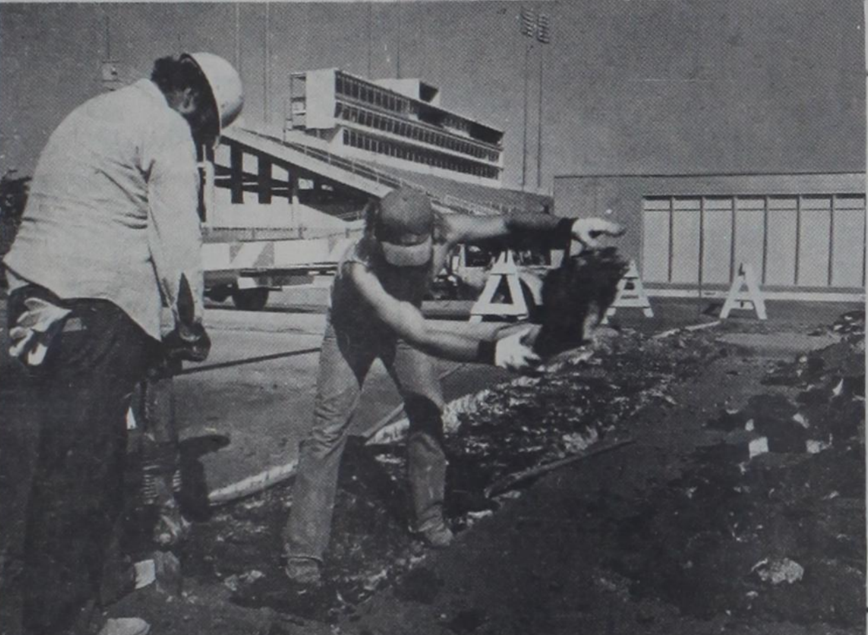
Workmen look for a broken sewer pipe at the 6th Street intersections Wednesday. Work on the street has caused a change in some of the bus routes on campus. (Photo by Max Faulkner).
