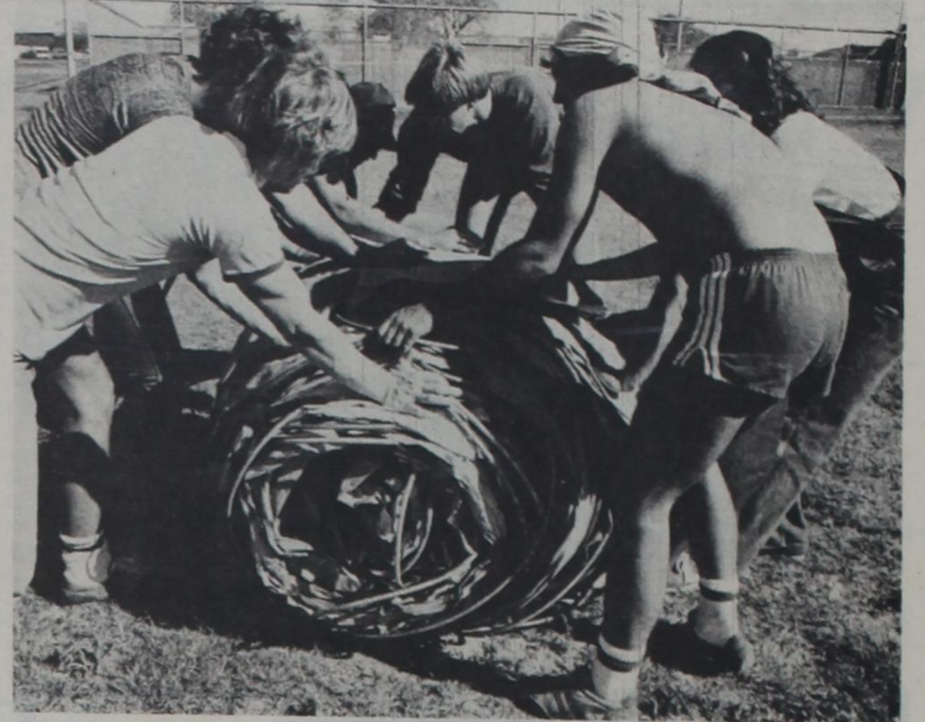
Members of Alpha Phi Omega unroll cables for the top of the Aquatic Center. The pool will be closed through Monday for repairs and replacement of the roof for the winter months. (Photo by Max Faulkner).
