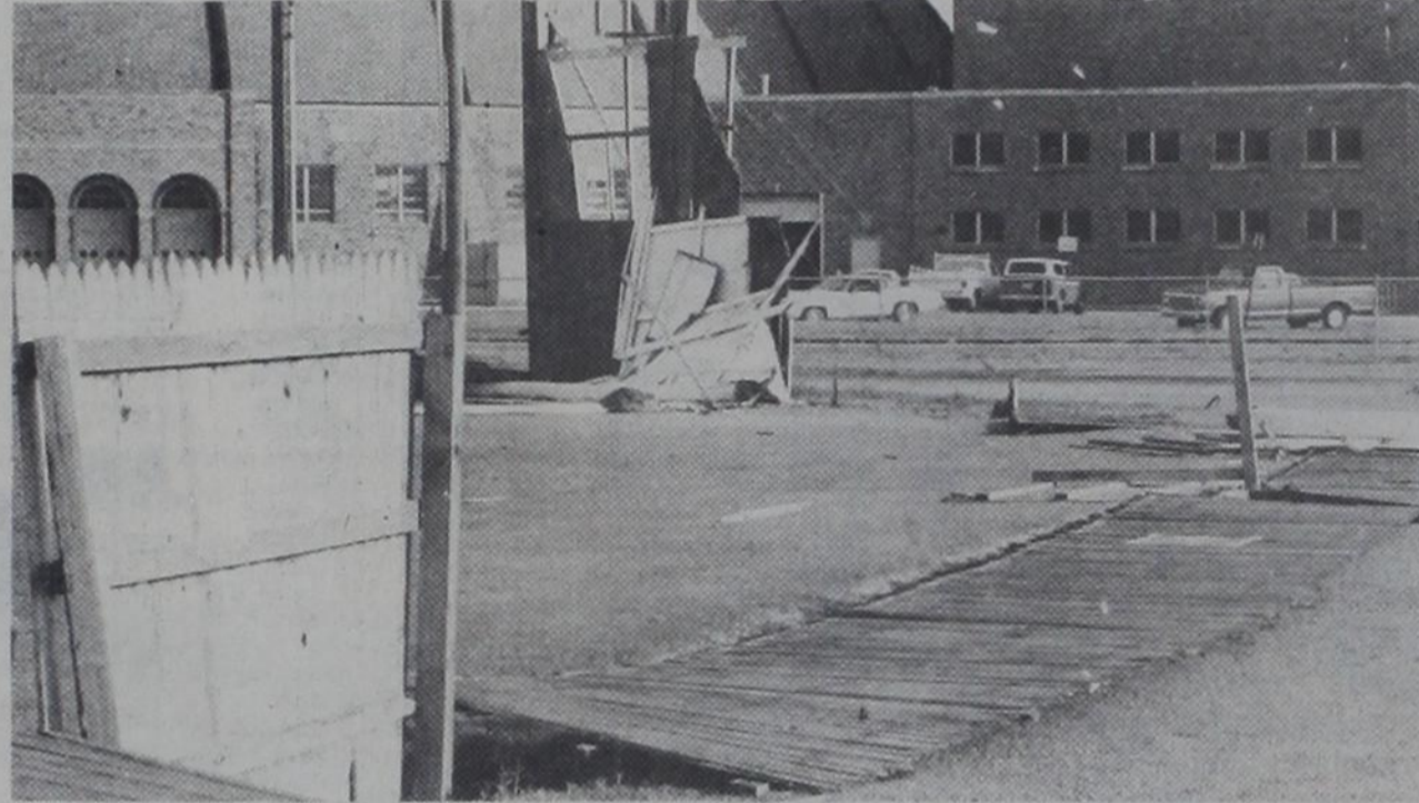
The scoreboard and fence at the Tech Sunday night's hurricane-strength wind baseball diamond lay on the ground after. (Photos by Ron Jenkins and Darrel Thomas)
