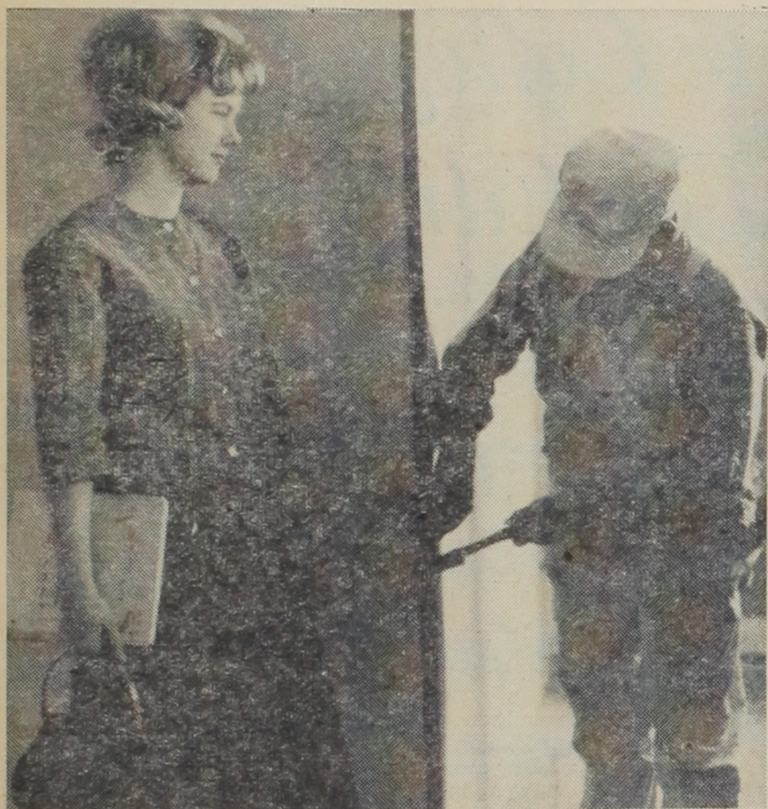
JUST CHECKING —Margie Bowling, Austin freshman, stops to give a little encouragement to a workman in the Social Science Bldg. which is being renovated. Construction is expected to be completed by March. —Staff Photo by Vernon Smith
