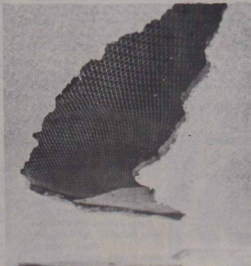
Damaged ceiling from water leaks
