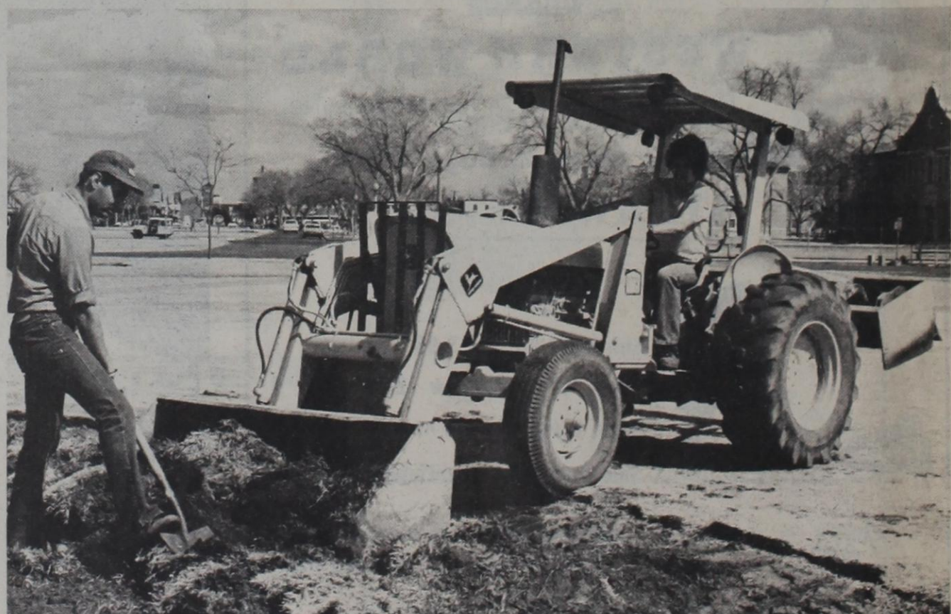
BEAUTIFICATION PREPARATION—Preparing grounds around Memorial Circle for landscaping are a couple of early season workers who are not exactly following the line of work they have chosen for careers. For instance, the tractor jockey is senior pre-dental major Bryan Itz of San Antonio and manning the shovel is history major Michael Christensen, Lubbock sophomore. (Photo by Debbie Elkins)
