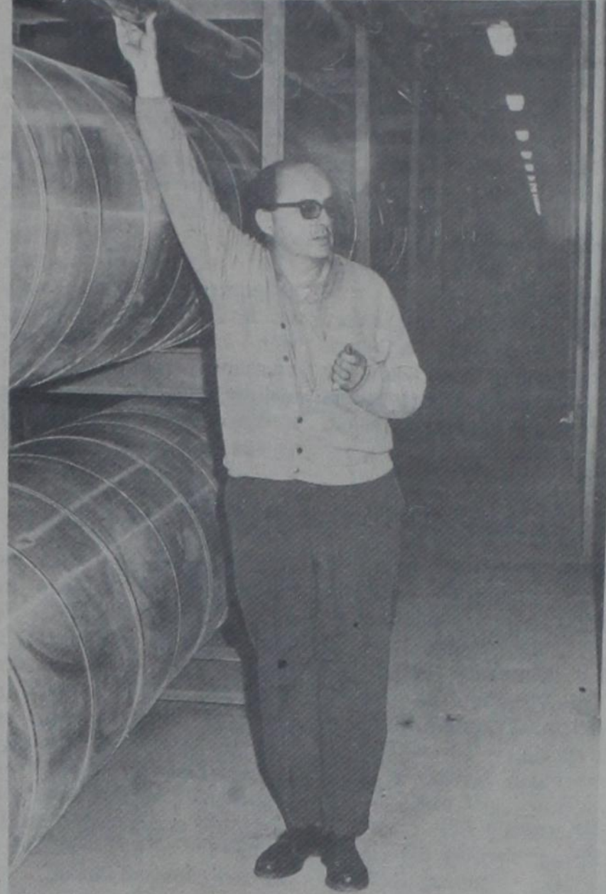
UD PHOTO BY KIM HITCHCOCK Paul Johnson describes purpose of pipes in tunnel system.
