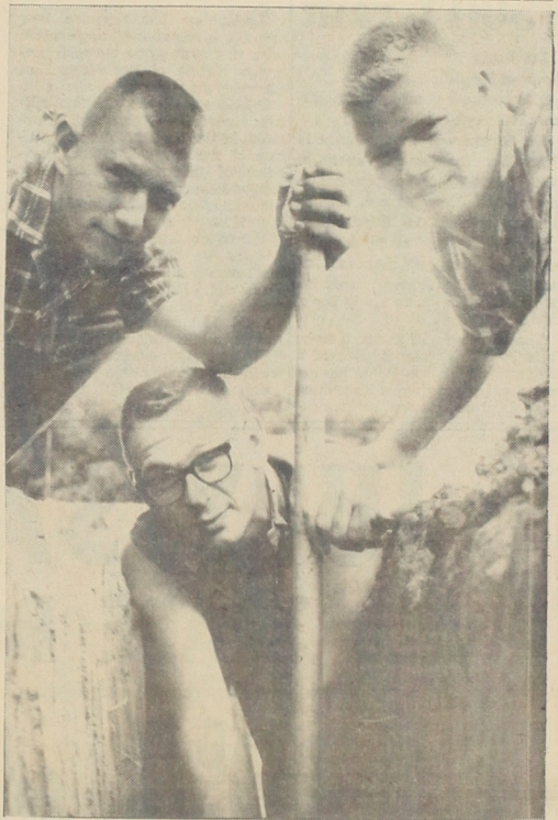
SUMMER MAINTENANCE —Pictured working on a pipeline for one of the women's residence halls—a part of the summer maintenance program underway on campus—are, left to right, Richard Garlitz, Bobby Overman and Roy Zickefoose. —Staff Photo
