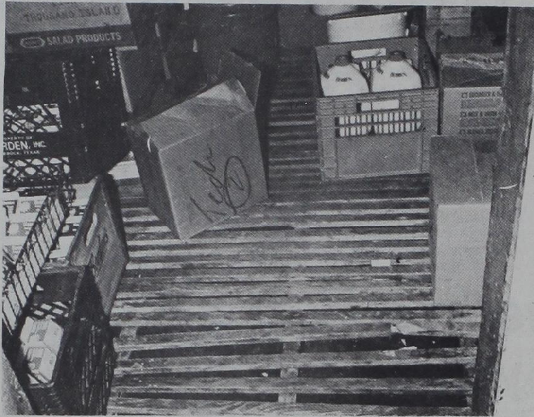
The photo above is the floor of one of the old refrigerators still in use in the UC. The refrigerators are too small and overcrowded to handle the increased demand for services. More money would allow a renovation of some facilities.
