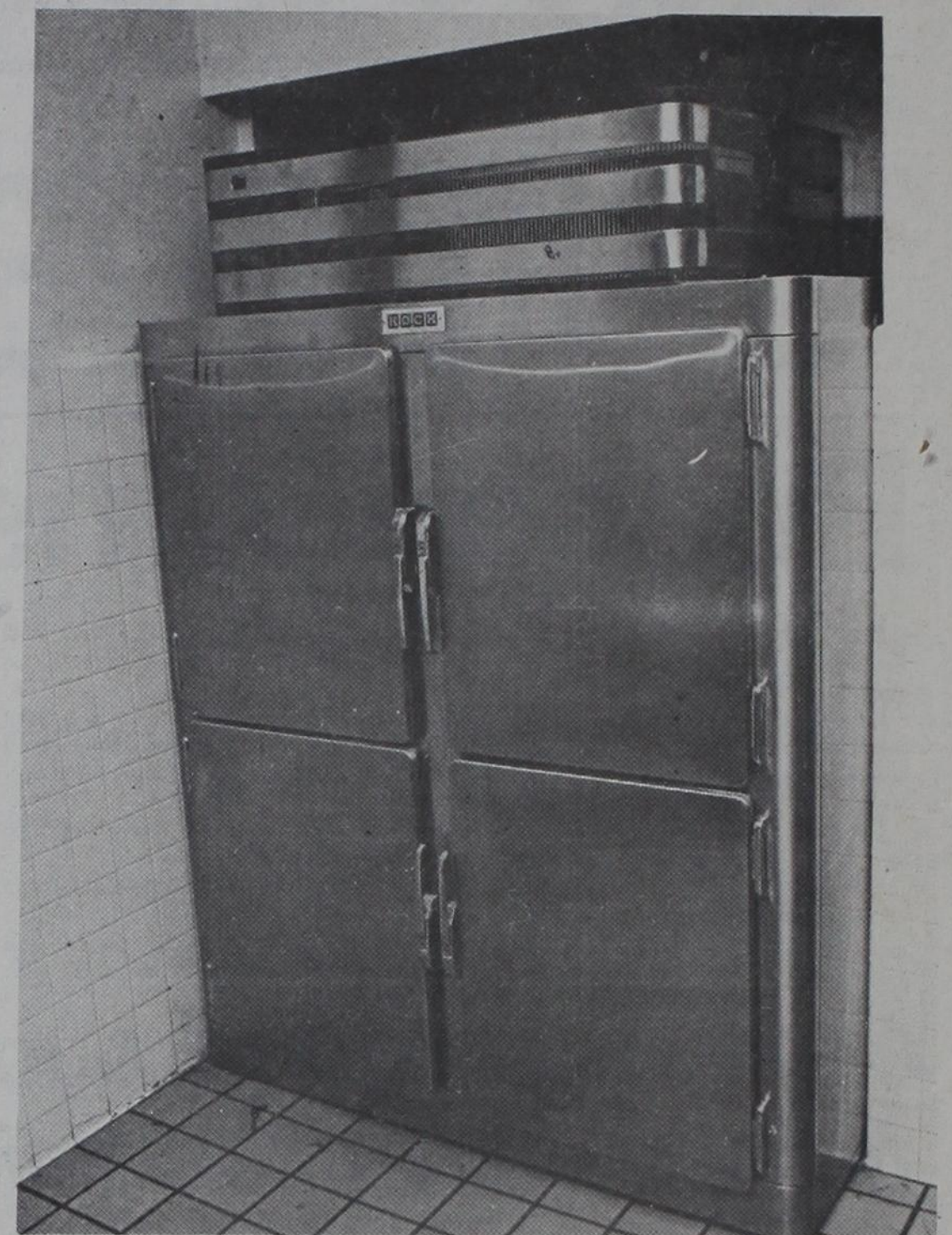
Lack of funds has kept this more than 20-year-old refrigerator in the UC even though it does not work. The machine is so old, parts can no longer be found to repair it. Because it was installed as a wall unit, it cannot be moved without leaving a large hole in the wall. (Photos by Mark Rogers)
