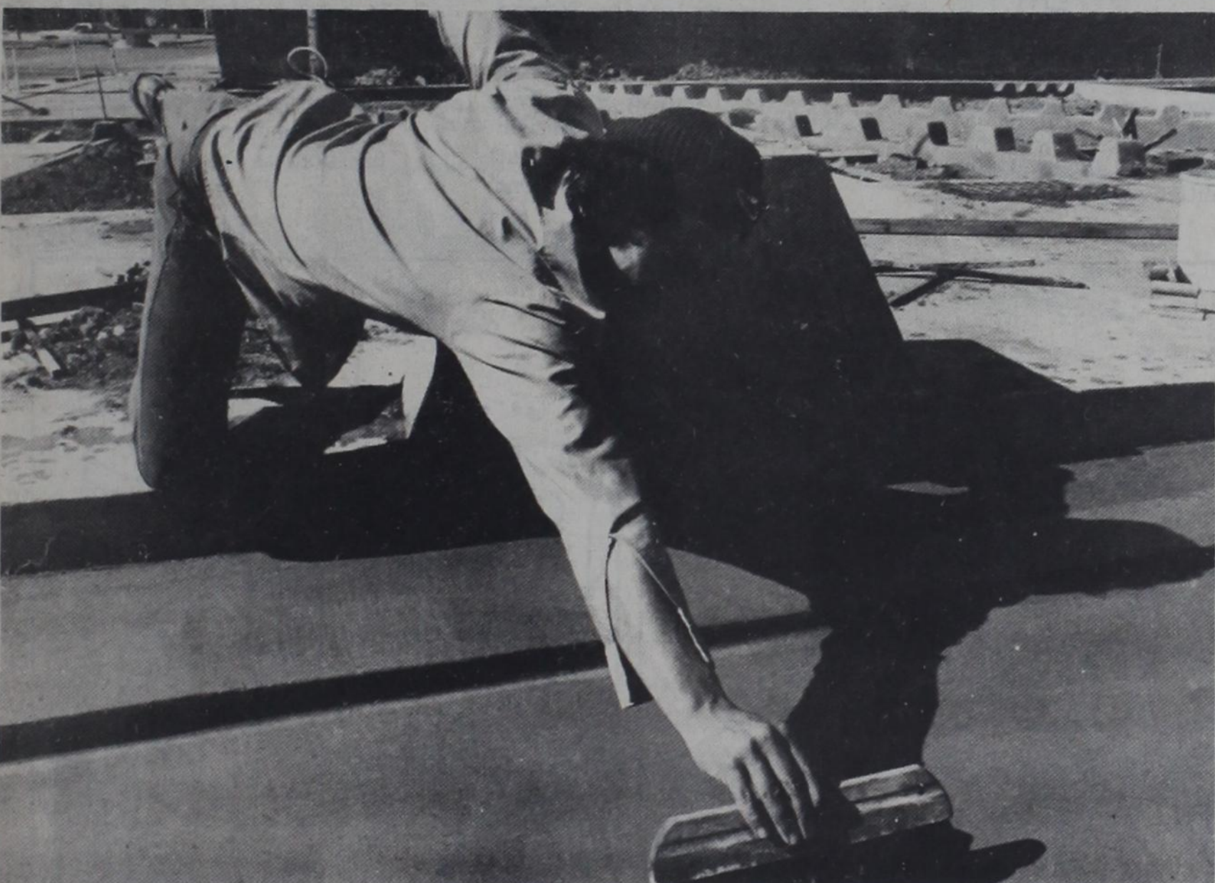
Albert Rodriguez smoothes out some concrete with his long reach at the construction site in the Doak parking lot behind the Tech bookstore. Construction has been taking place all over campus as a sign that the Tech campus is growing. (Photo by Mark Rogers)
