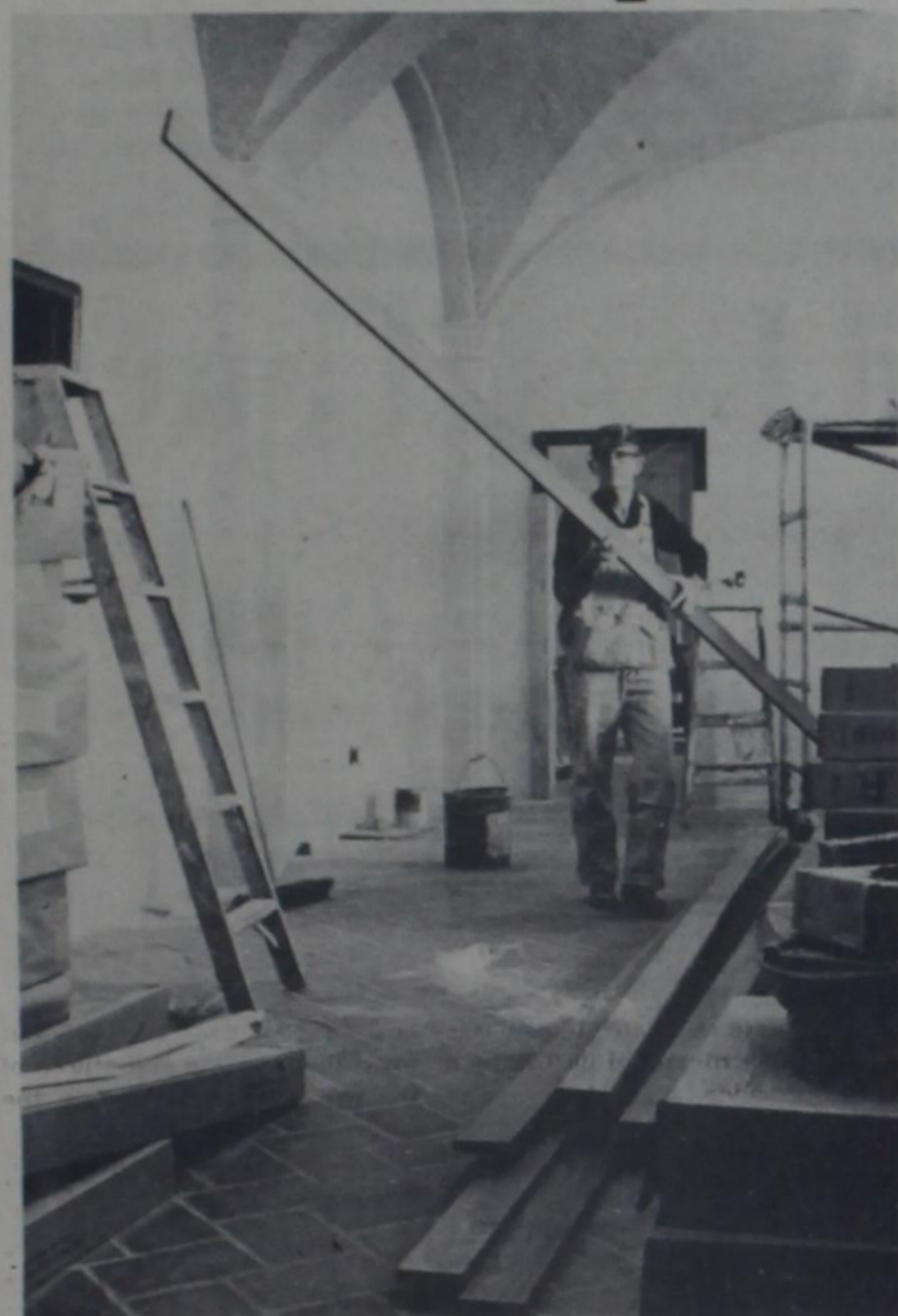
Workmen continue to remodel offices in the east wing of the administration building.
