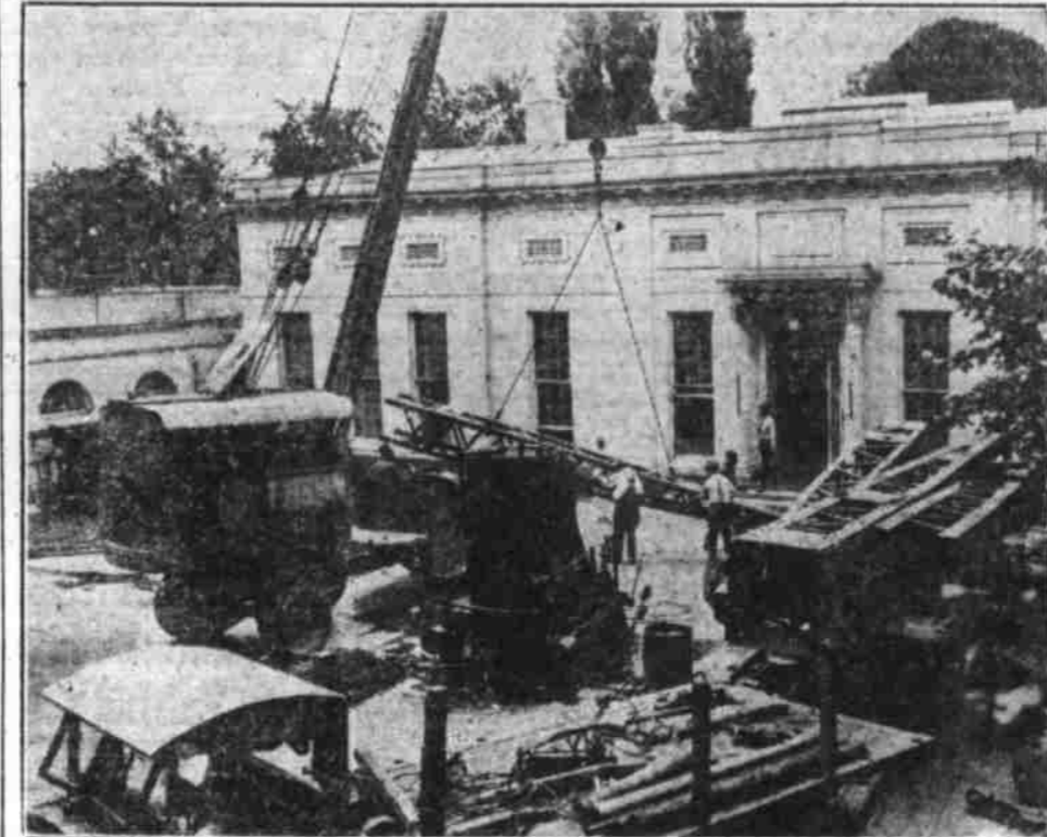
The task of enlarging President Roosevelt's office in the White House has been started. Workmen are shown as they arrived on the scene with cranes, trucks and other implements. The project is to cost $303,087. The executive office was built during the administration of Theodore Roosevelt. (Associated Press Photo)
