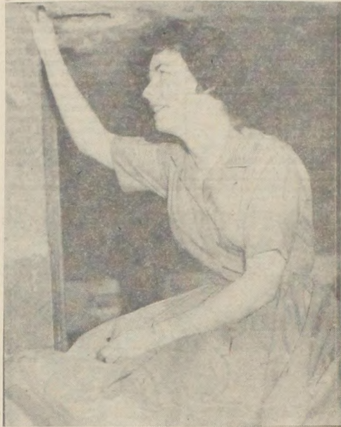
APPREHENSIVE — Mollie Sue Wallace, sophomore journalism major from Waxahachie, found a comfortable place to sit Friday afternoon — underneath 380 tons of concrete! The east roof section of the new classroom and office building had been raised about 37 inches as Miss Wallace steadied her nerves and perched beneath the slab.
