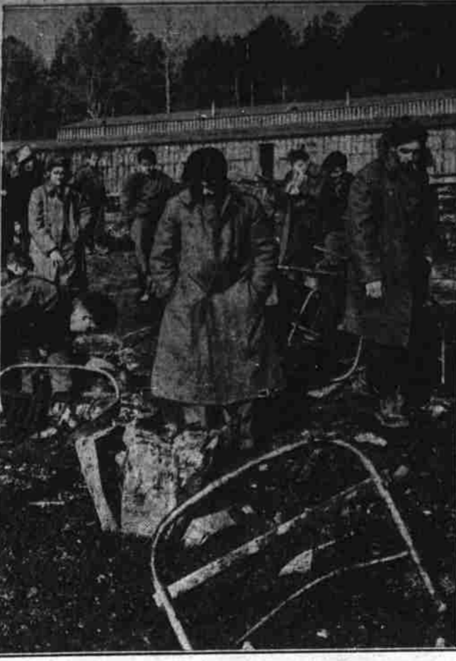
Army officers at Norris, Tenn., began an investigation of the fire which destroyed three barracks of a CCC camp near there, burning three boys to death and leaving four suffering from burns. CCC workers are shown inspecting damage done by the blaze. (Associated Press Photo)
