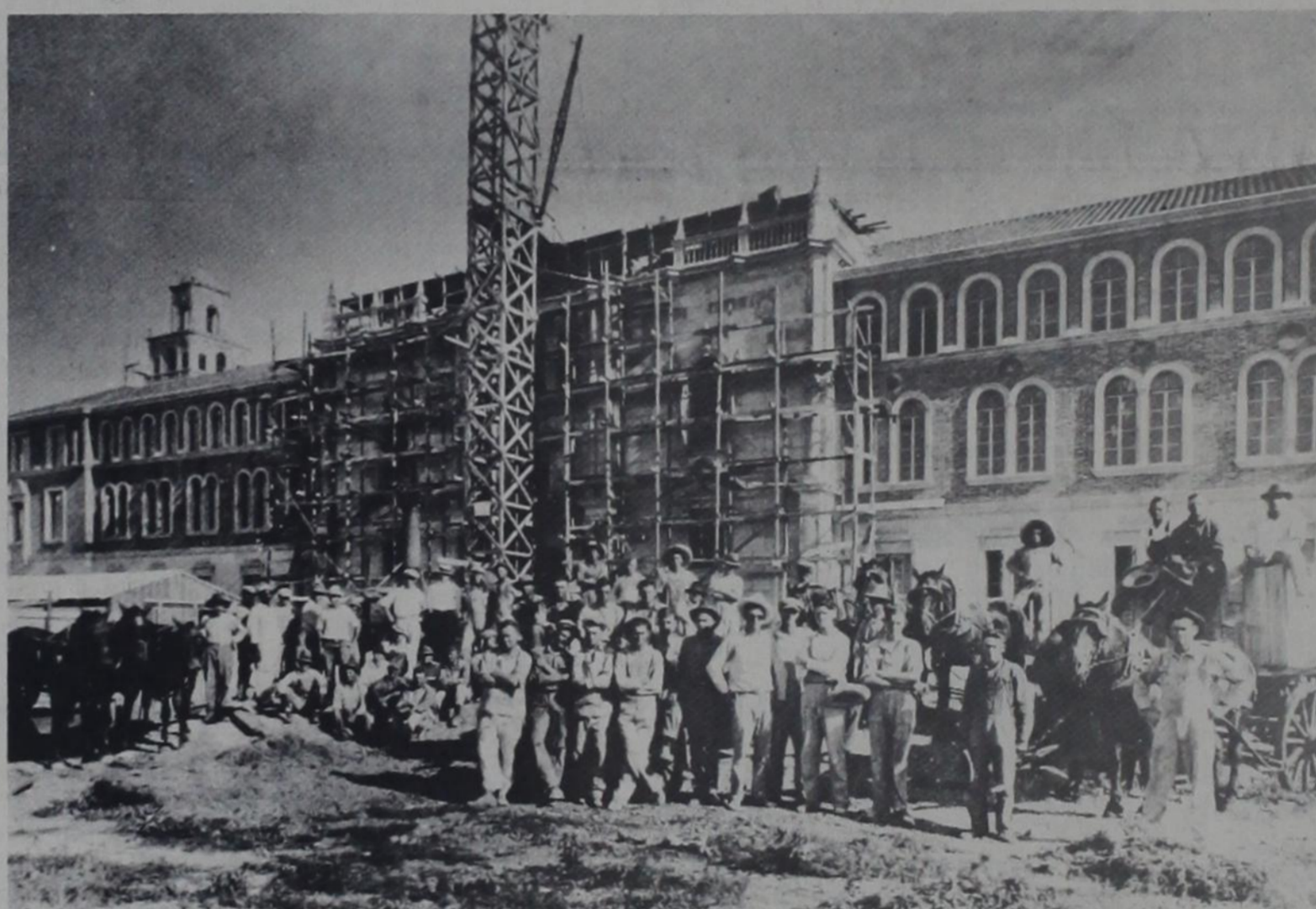
BUILDING CREW — Several men working on the Administration Building take time out to pose for pictures. Horses and wagons were used in the early construction.
