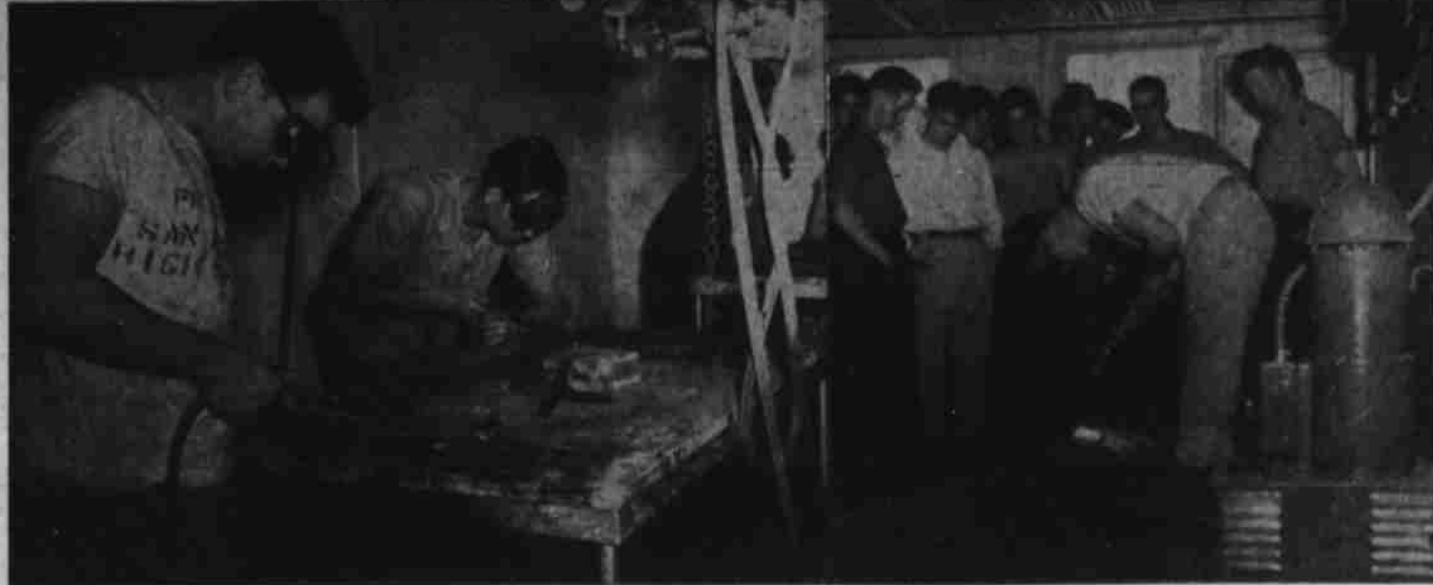
Playing With Fire? Well, hardly, for these young men are learning to work with it as they put into practice instructions in welding as afforded in the national defense class sponsored by the Big Spring Independent school district in cooperation with the vocational education unit of the state department of education and the federal government. Left, two NYA enrollees meticulously practice on patch work while (right) several gather around while one uses the acetylene torch to cut cut sheet steel for the work. There are three classes offered, those for NYA lads, those out-of-school youths, and for experienced men taking a "refresher" course. (Ferry Photos)
