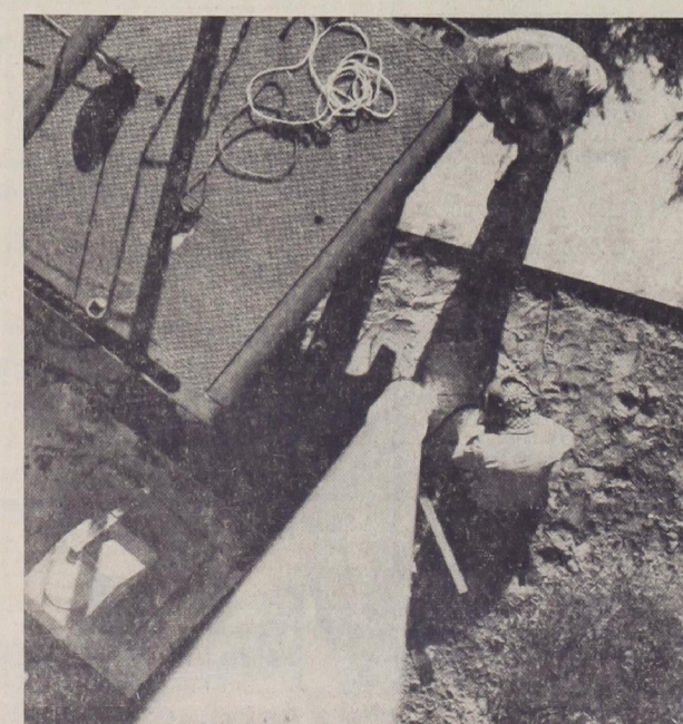
ROOM AT THE TOP? —University Daily Photographer Johnny Shipman captured this flagpole sitter's view of the flagpole being installed in Memorial Circle. Shipman shimmied up the winch of the workmen's truck and dangled precariously to click the shot.
