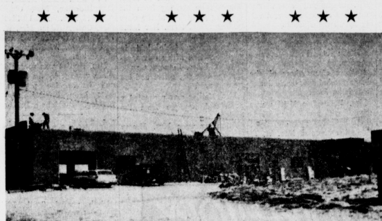
AG BUILDING SPEEDS - The new structure just west of the swimming pool has reached the roofing stage to make it one of the most advanced of all the building projects. This structure will be used for shops.
