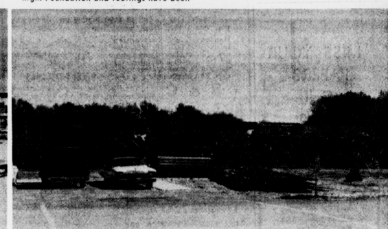
CLASSROOMS - Junior high school is to have an addition to both ends of the present building. Here's the classroom addition which has reached the brick-laying stage.
