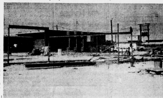
CAFETERIA STARTS - Floors and foundation have been laid for the new 650-seat junior-senior cafeteria, and this past week workmen started putting up the steel framework.
