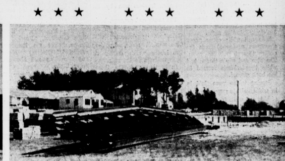
GYMNASIUM - Among the additions planned is a new gymnasium for junior high. Foundation and footings have been run, and steel and brick were being moved in last week.
