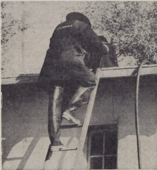
CAMPUS FIRE—A Lubbock fireman climbs the roof of the sculpture kiln, located north of the Architecture Building, to extinguish a fire Wednesday which did approximately $200 damage to the structure.
