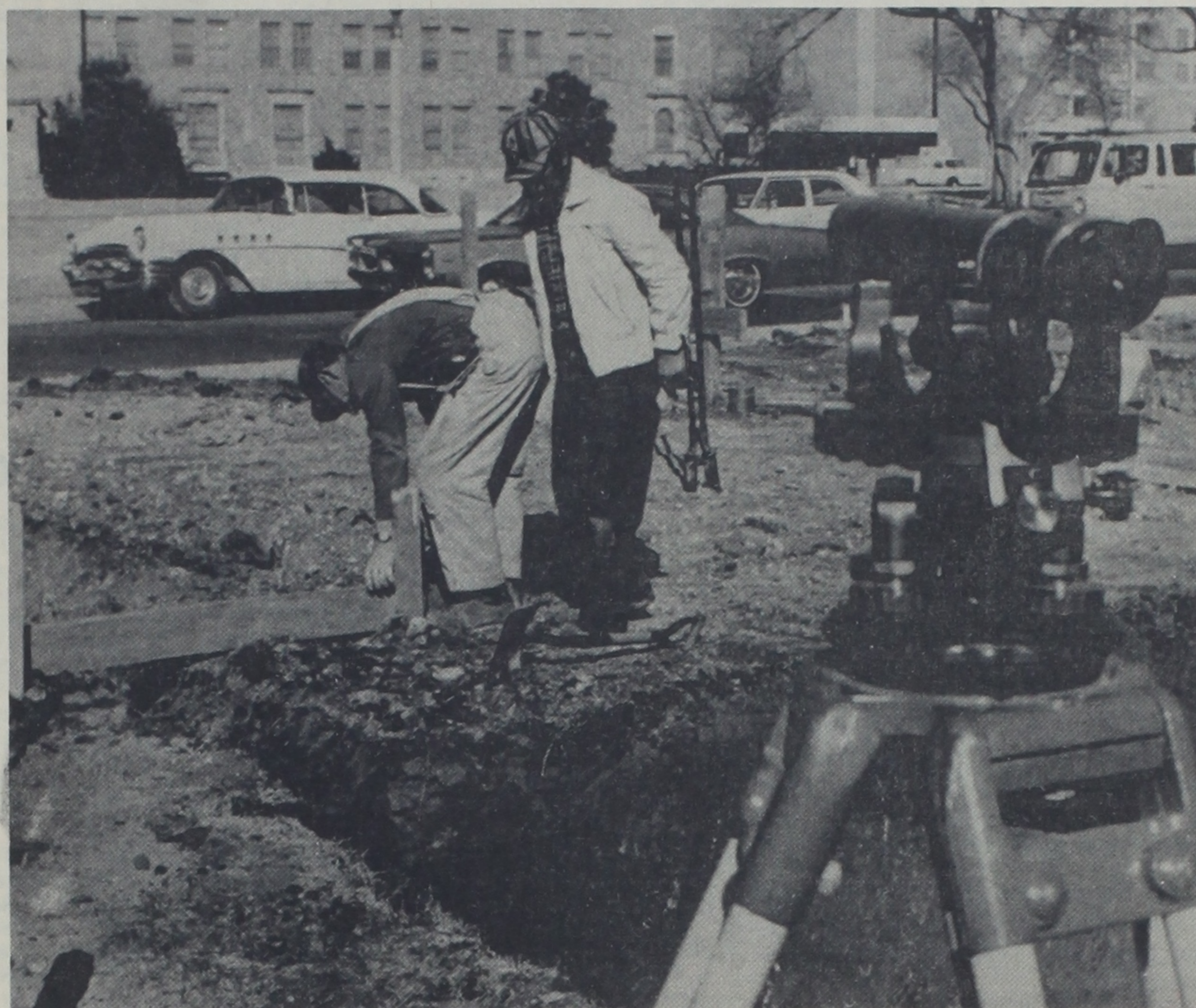
COMMENCEMENT EXERCISES—Work has now commenced on the Amon G. Carter Plaza, long-awaited entrance marker for the campus at the Broadway en-
