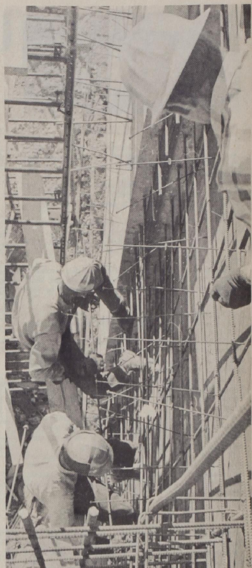
MONEY SQUEEZE — Federal cuts in education spending have severely curtailed construction on college and university campuses, such as that now in progress at Tech's new building for the School of Business Administration, and have forced institutions to use fees for badly needed revenues.
