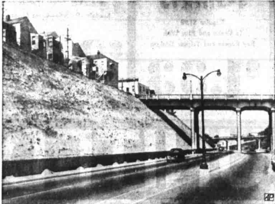
CONCRETE SOLUTION —Wall of Bernal Cut, San Francisco, Cal., once a source of danger on account of minor rock slides, lets loose no more since it was sprayed with cement.
