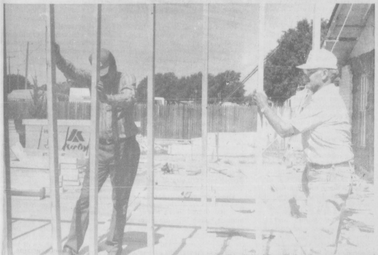
John Brown [left] and Raymond Birchfield assist with the building project at the Primera Mission Bautista.
