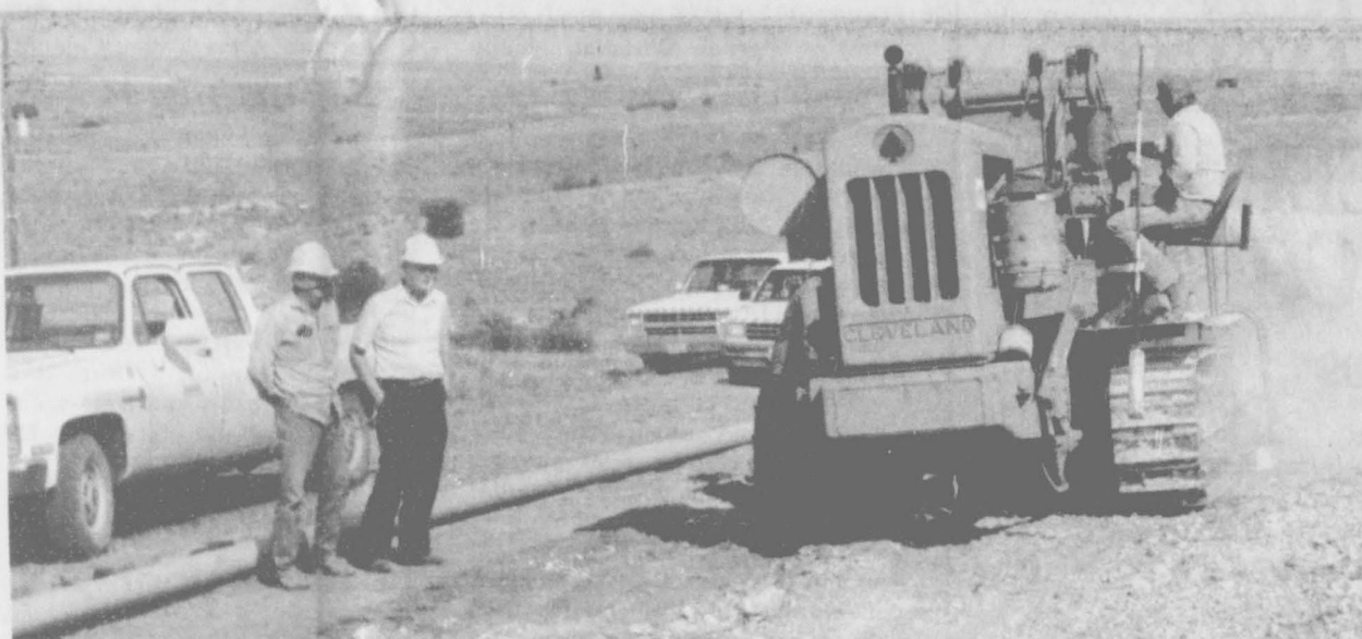
Beginning the advance preparation for the dam project, these men are moving pipelines so the boundaries for the dam project will be in order. Working for Natural Gas Pipeline, Joe Ellison [left] is welding inspector, and Charles Little [center] is foreman for Natural, supervising the moving of the pipeline. George Ford [right] is working for Energas Construction and doing the actual moving of the pipelines.
