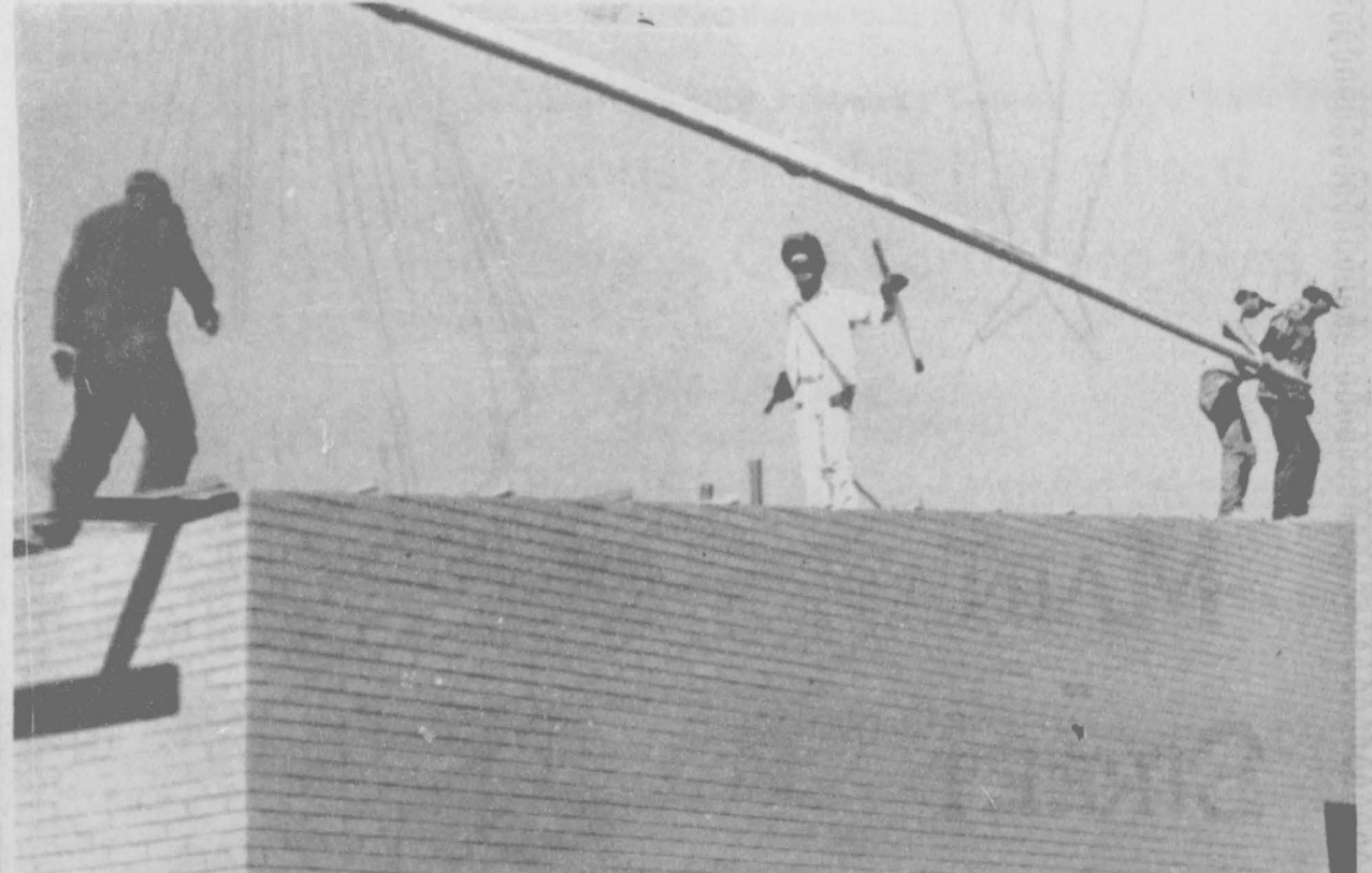
Standing on the edge of the roof, these workers at the Spearman Elementary School are putting some finishing touches for the awning work on the roof before they get the rest of the weekend off to enjoy the Thanksgiving Holidays. The job superintendent
