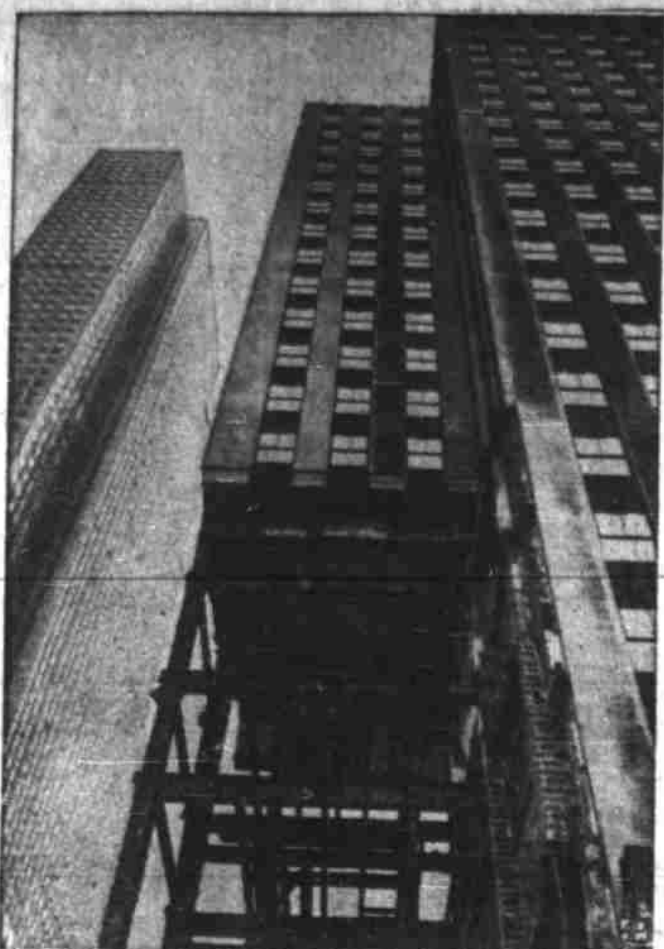
SKYSCRAPER ON STILTS —Upper floors of the U. S. Rubber building in New York's Rockefeller Center rest on steel girders bared by the demolition of the Center Theater. The latter, ripped out of a lower corner of the building, will be replaced by office floors. The RCA building is at left. View is from Avenue of the Americas.
