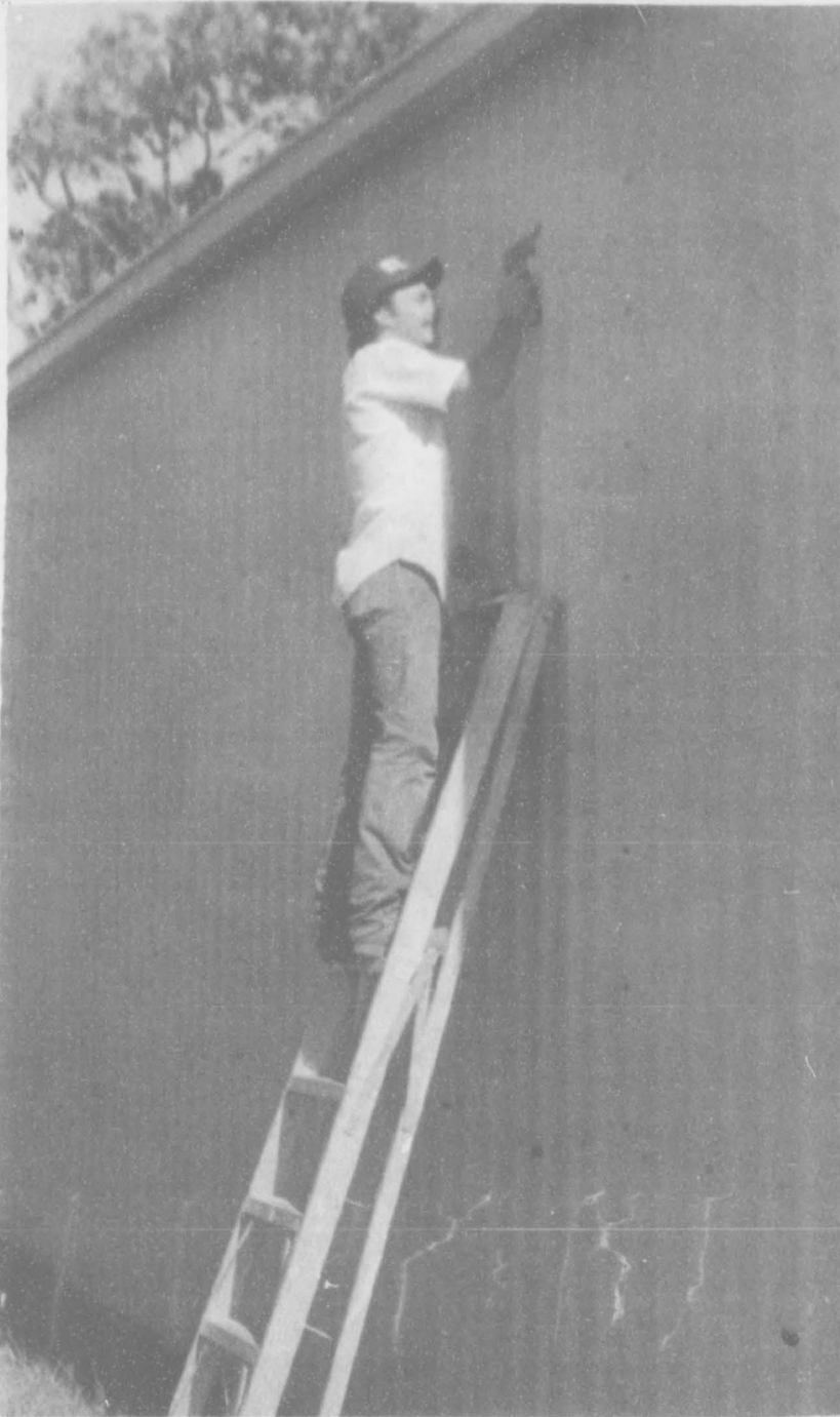
OK, sir, were you really smiling before I got the camera out? This young man [Clint Sanders] is sanding the Golden Spread Senior Citizen Building preparing it for a new paint job. Jim Beasley's Construction has been contracted to give the Center it's new face lift.
