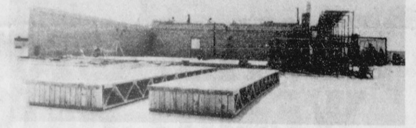
Progress is being made on the new 1st National Bank in Spearman. Girders for the roof have arrived and three of the four walls
