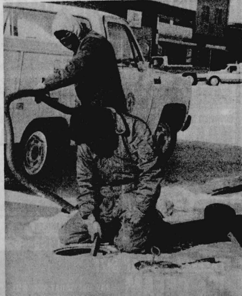
A cold necessary job—on Dec. 29, one of the colder mornings of the year, City of Spearman employees Walter Esquebel [kneeling] and Leo
