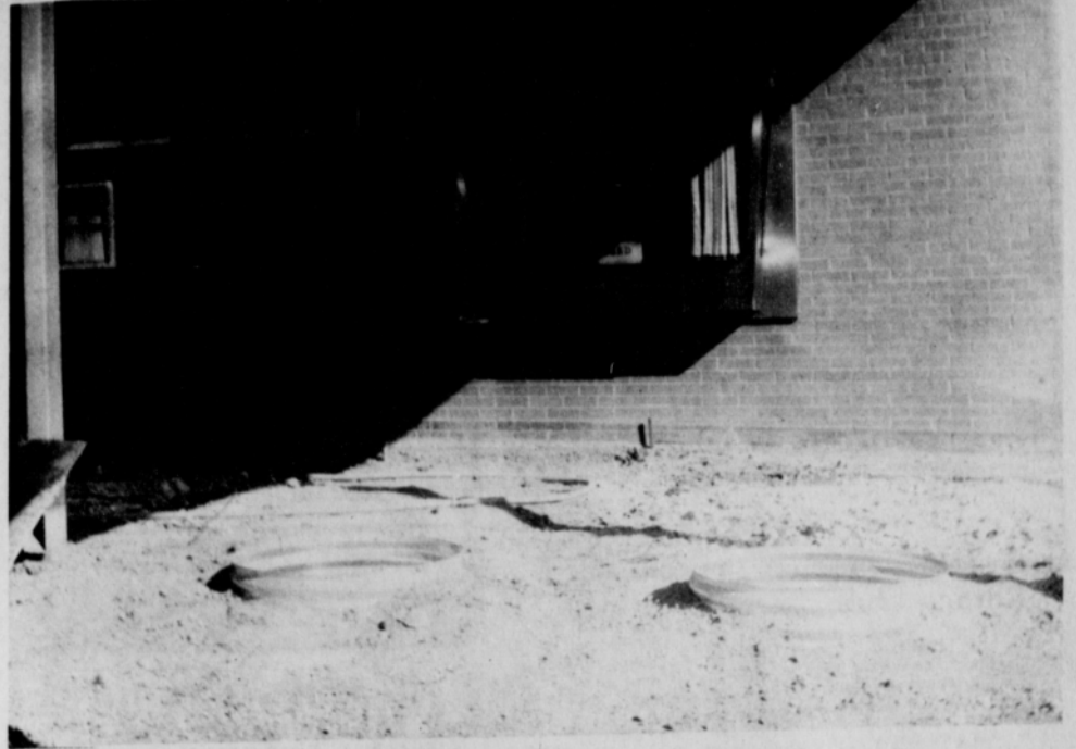
The drive up window at the First State Bank has been closed for quite some time, but in the near future, patrons will have two windows to use. Notice the two large holes in foreground, site of the new drive up window.
