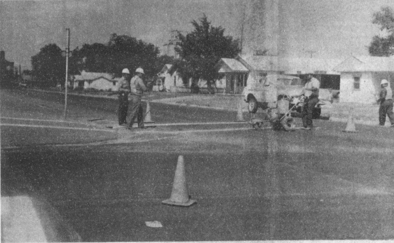
GETTING READY FOR SCHOOL --City workers have been very busy the past several days, striping crosswalks around the local schools, especially the two elementary schools, where hundreds of students will be crossing in the next couple of weeks when school starts again, September 3. Law enforcement officers and school officials are asking all motorists to be very aware that school time is near.
