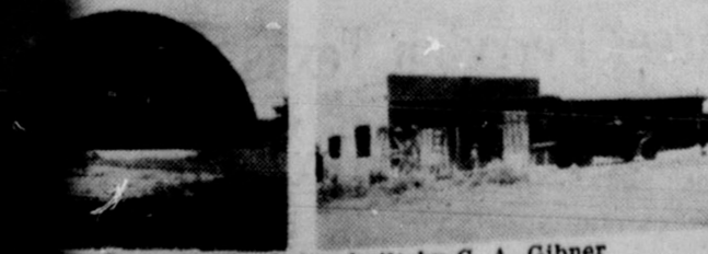
Quonset Hut being built by C. A. Gibner Super Service Station Under Construction
