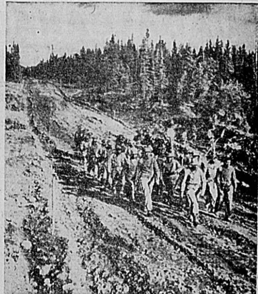
DAY BY DAY, MILE BY MILE —A ribbon of civilization through the wilderness of Northern Canada and Alaska, the Alcan Highway linking U. S. and Alaskan outposts, a dream of but a few years ago, is in final construction stages. U. S. Army labor battalion trudges back to camp after another day of toil.
