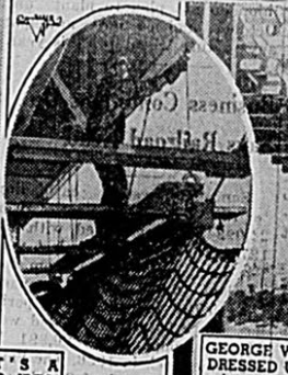
GEORGE WASHINGTON BRIDGE BEING DRESSED UP —Safeguarded by rope-line a large squad of painters scramble every morning over the railing to the scaffolding below. The repainting of aluminum color in keeping with the rest of the span is a continuous process with a different section scheduled each year. It is not unusual for the George Washington Bridge and Holland Tunnel to pay the 50,000 mark on Sunday.
