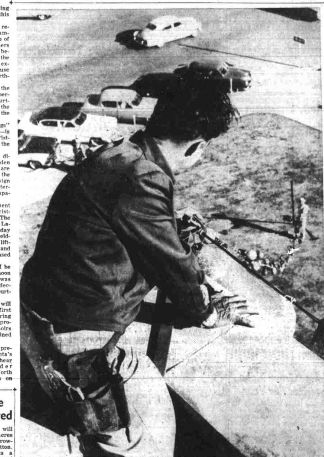
CHRISTMAS LIGHTS GOING UP . . . OR DOWN Sig Rogers and helper stretch streamer from courthouse roof
