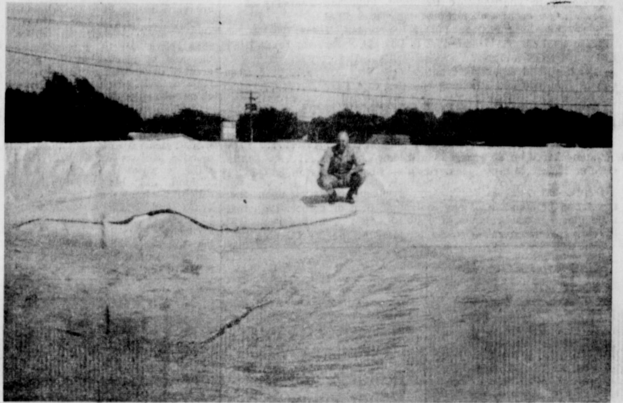
E. J. COPELAND is pictured on top of the Equity store house, beside the large hole in the roof, caused from the heavy rains over the week-end. Rainwater caved in the roof, and damaged a large part of the Equity seed and feed stock.
